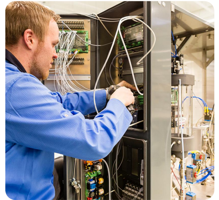
System integration at Sieradz plant in Poland.
